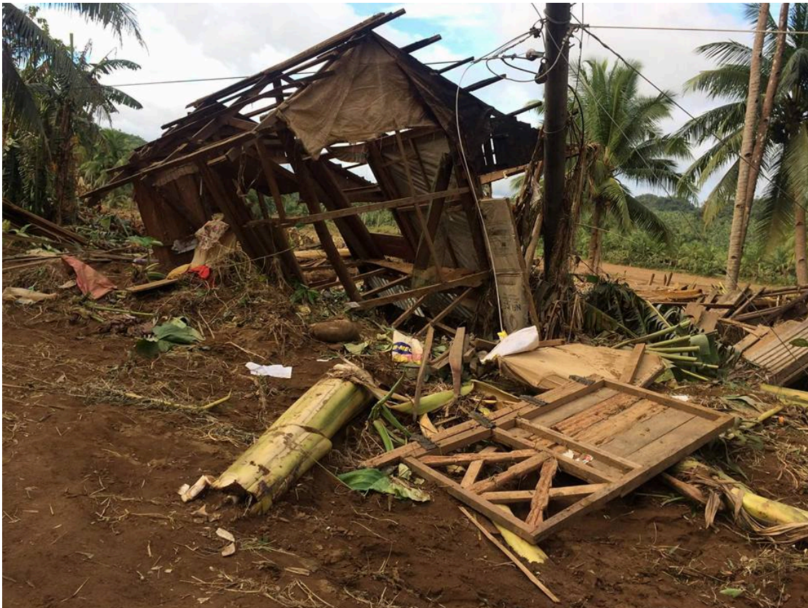
Totally-damaged house in Borongan, Eastern Samar. (photo credit: LCDE)
