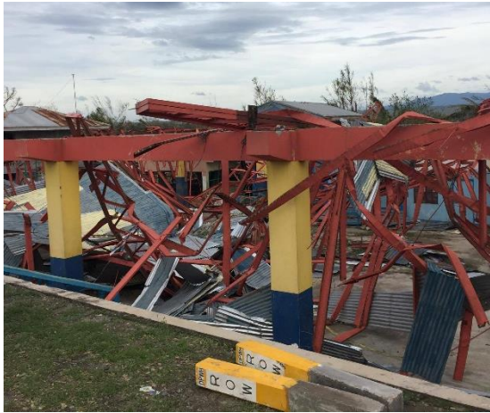
Collapsed structure due to typhoon Karen
