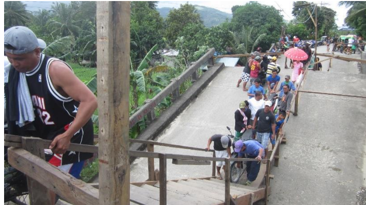
Collapsed bridge in Surigao City after the 6.7 magnitude earthquake
